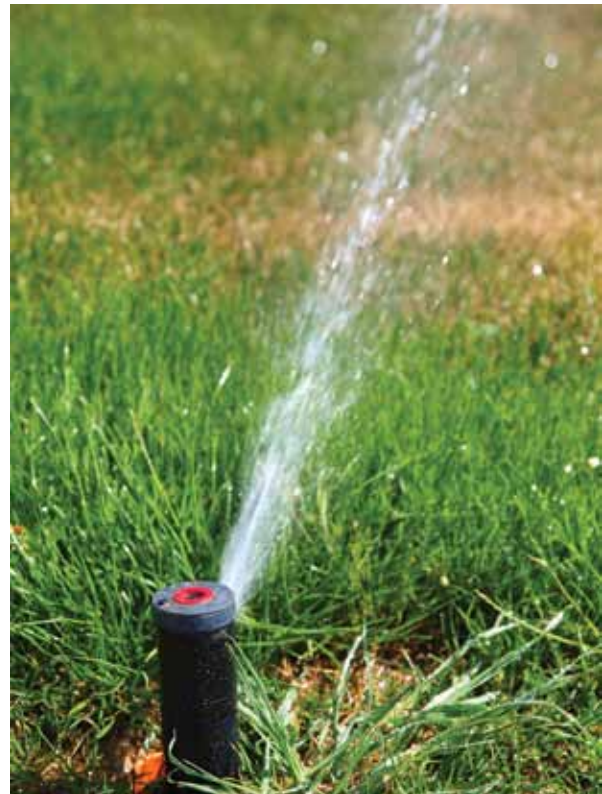
Many communities have passed water conservation ordinances that include, among other things, irrigation methods and timing.
